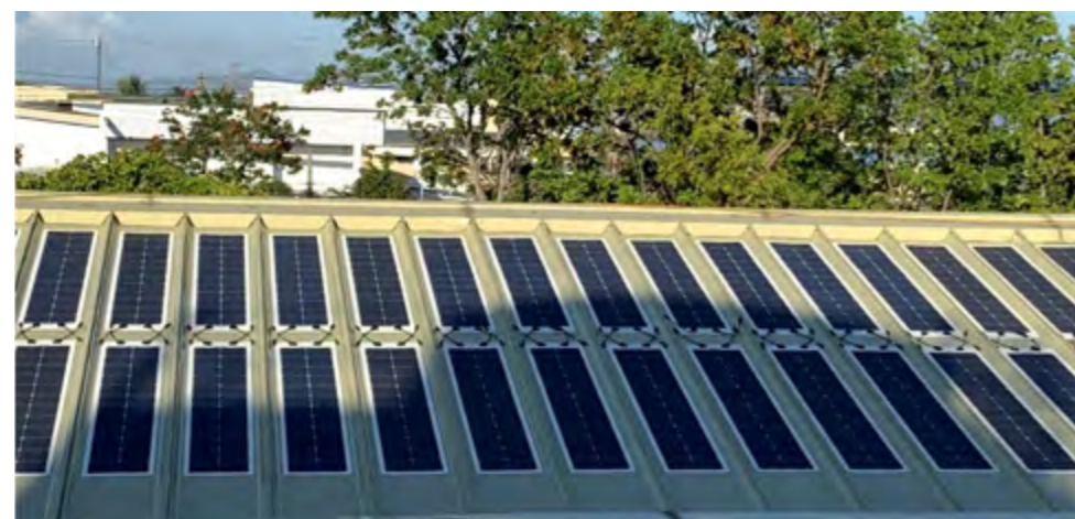
IMI's Solar Pilot Project Initiative using Merlin® Solar's Patented Technology, has generated 10.8 Megawatt hours of clean and renewable energy source from the sun, powering the Air Conditioning System of the building's cafeteria. This system has its contribution in the reduction of carbon footprint and greenhouse gases, equivalent to around 10,155 kilogram (10Tons) of CO 2 emission.
