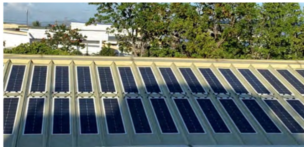
IMI's Solar Pilot Project Initiative using Merlin® Solar's Patented Technology, has generated 10.8 Megawatt hours of clean and renewable energy source from the sun, powering the Air Conditioning System of the building's cafeteria. This system has its contribution in the reduction of carbon footprint and greenhouse gases, equivalent to around 10,155 kilogram (10Tons) of CO 2 emission.
