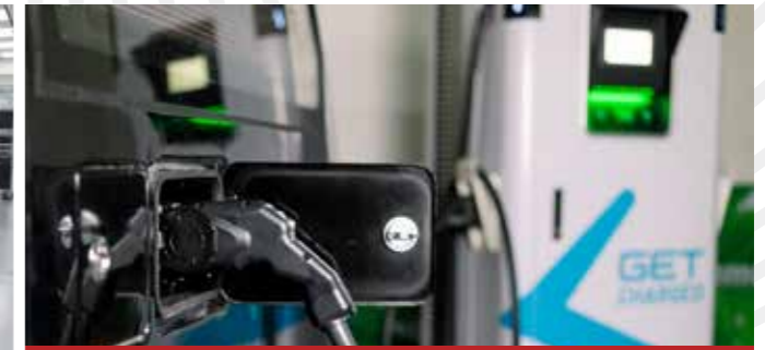
IMI brought EV chargers to the Philippines; the 1st integrated EV charging & transport system for the Ayala group was installed in December 2021
